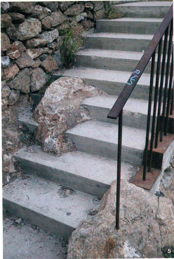
5 Turó de la Rovira is the remains of an anti-aircraft embattlement, and then a shanty town, in Barcelona by architects AAUP + JDVDP. Photo: Billy Maynard.
